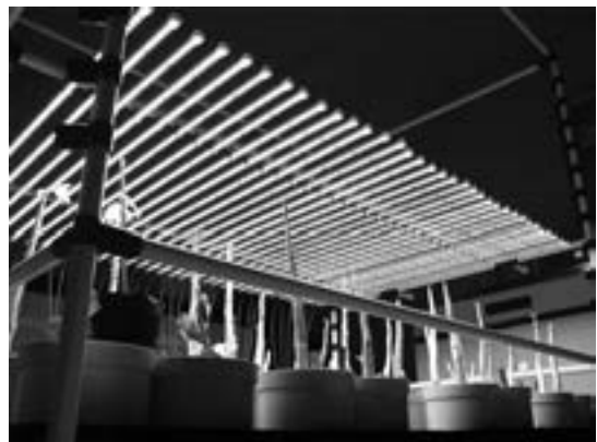
LED lighting system for tree plants.
