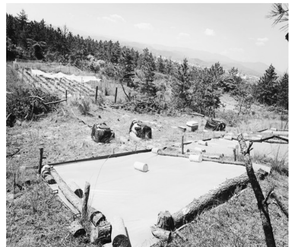
An experiment for water harvesting system with a plastic sheet and a tank in ALRC
