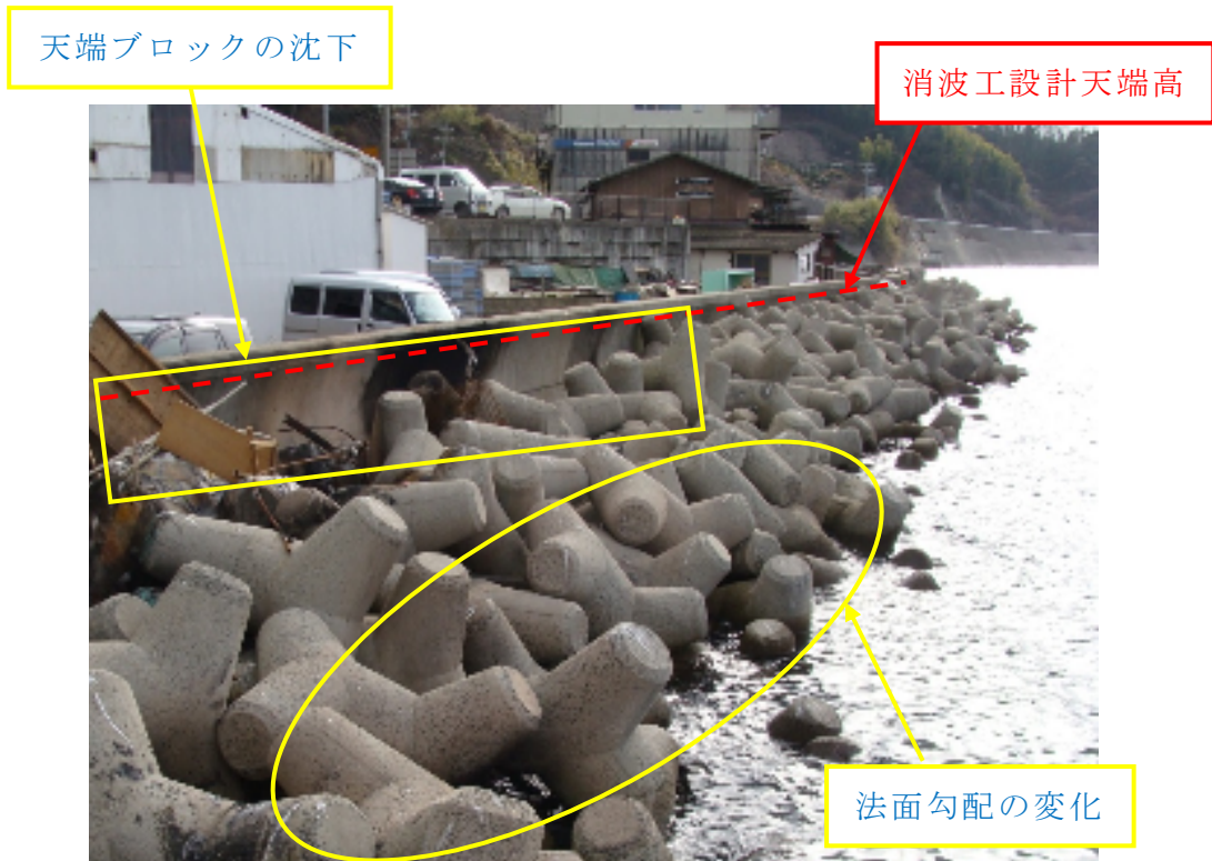
(護岸消波工の被災例)
