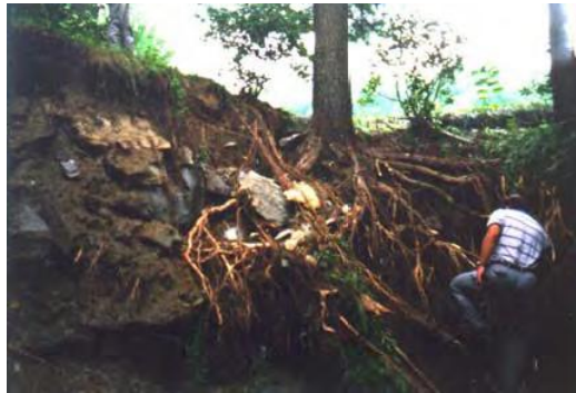
Fig.2.5. Tree root induced scouring on crest and downstream face[6]
