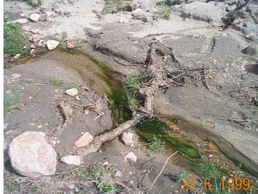
Fig.2.3. Dam failure due to root penetration in Colorado[6]
