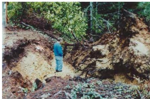
Fig.2.2. Serious damage by uprooted tree to embankment stability at a dam in Oregon[6]
