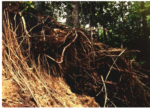
Fig.2.4. Exposed tree roots in overtopped dam[6]
