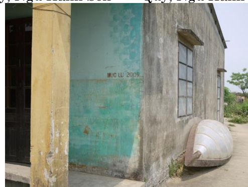
Flood mark in house's wall - Cam Le
