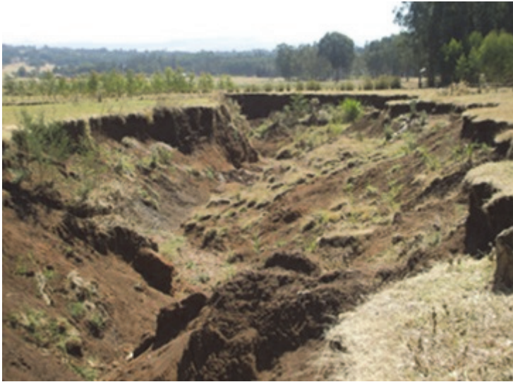
Figure 6. Evidence of active gully-head and -bank erosion in northwest Ethiopia (maximum depth = 1.5 m).
