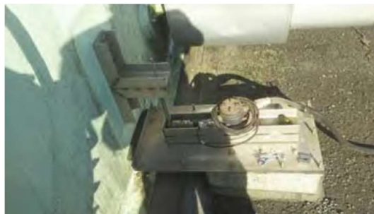
Figure 1.20 Spring-Operated Displacement Gauge Placed at Bottom Part of Shell Plate of 115,000 kL Capacity Tank [24]
