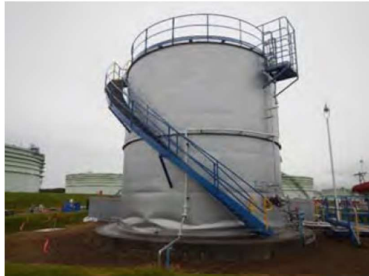
Figure 1.19 Buckled Shell Plate of 306 kL Capacity Bunker Tank [24]
